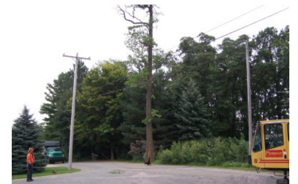
Picture 4: Crane lowering tree near power lines
